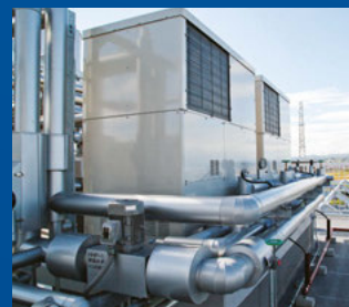
Emergency-ready Gas cogeneration
