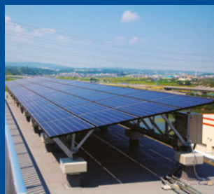
Solar power generation panel
